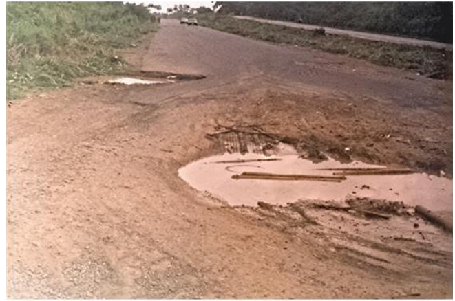
PLATE 2: Dangerous potholes, Lagos-Ibadan Expressway, Nigeria
