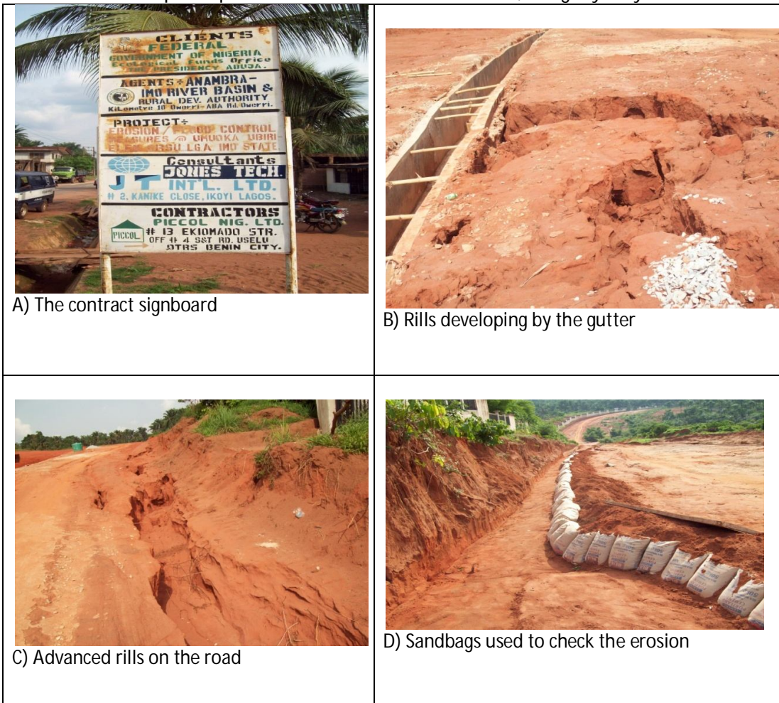
Figure 3: Umuoka Ubiri Elem erosion site
